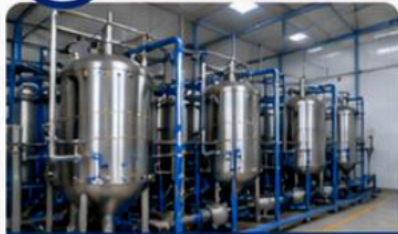
Sistem Filtrasi & Water Treatment
